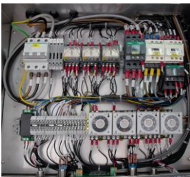
Movable electrical box
